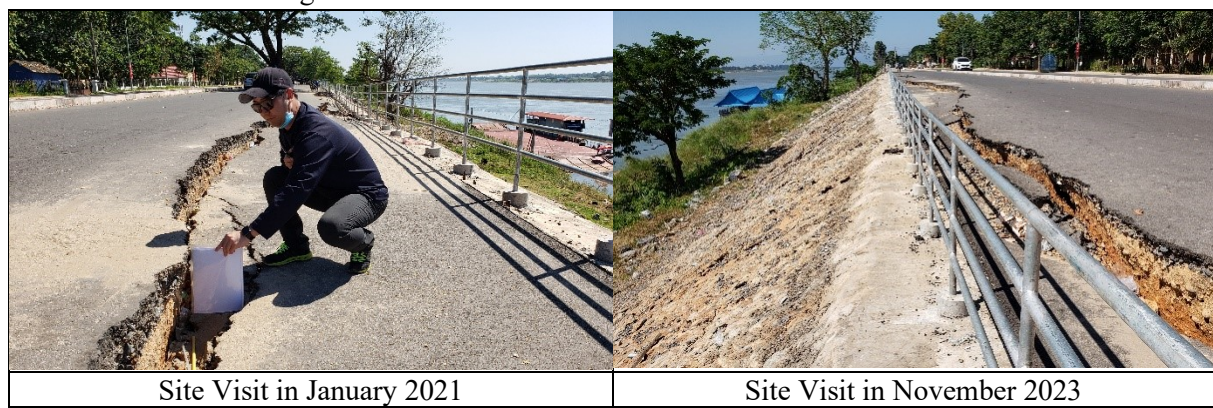
Figure A1-1 Ongoing Crack on the Riverside Road
