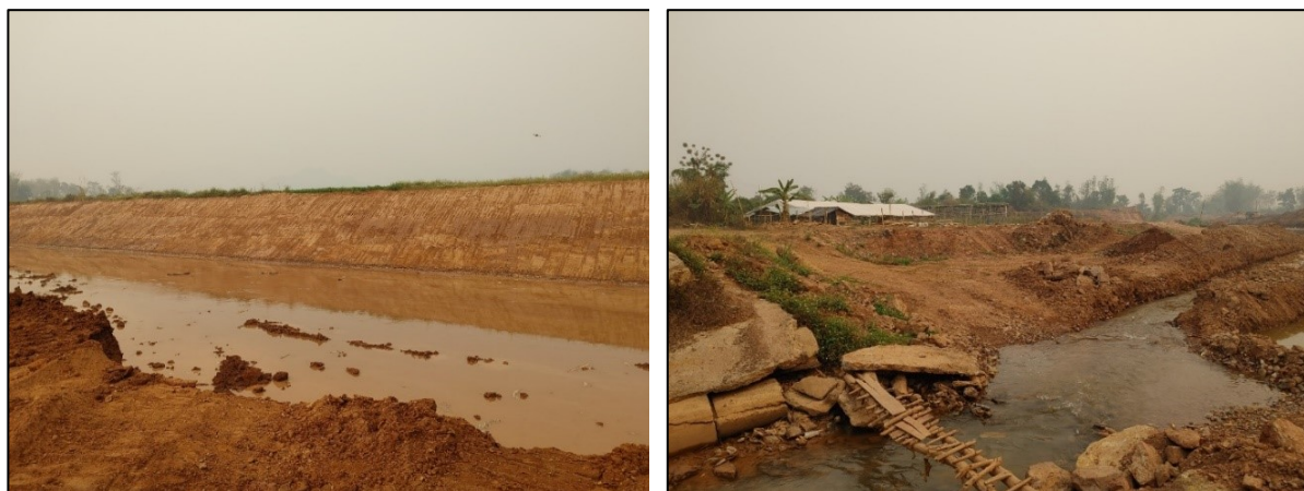
Figure A1-2 Excavated Riverbank Condition at the Left Side of the Nam Mao River
