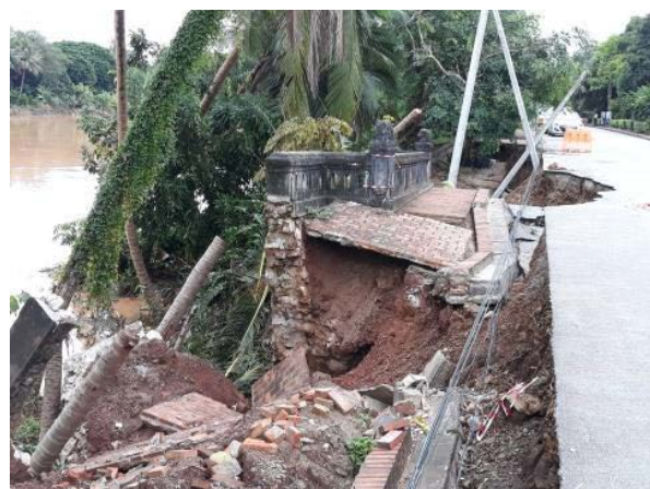
Damage of Son-Tinh tropical storm on the Nak Khan riverbank (accredited: World Heritage Office, LPB)
