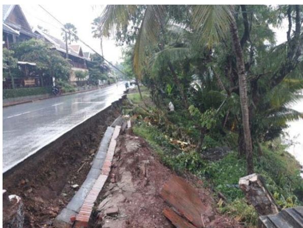
Damage of Son-Tinh tropical storm on the Nam Khan riverbank (accredited: World Heritage Office, LPB)
