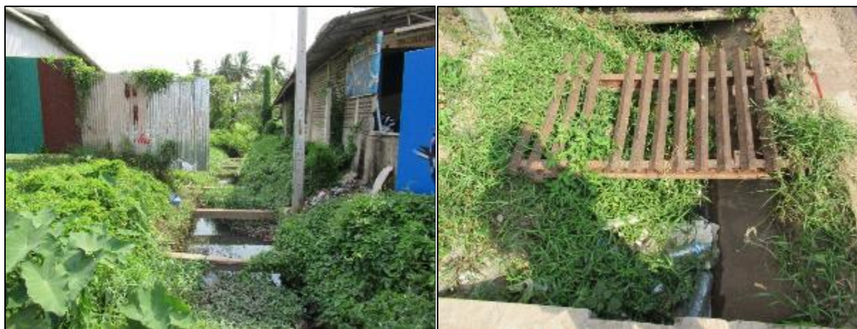
Figure 12: Example of Poorly Maintained Local Drainage System
