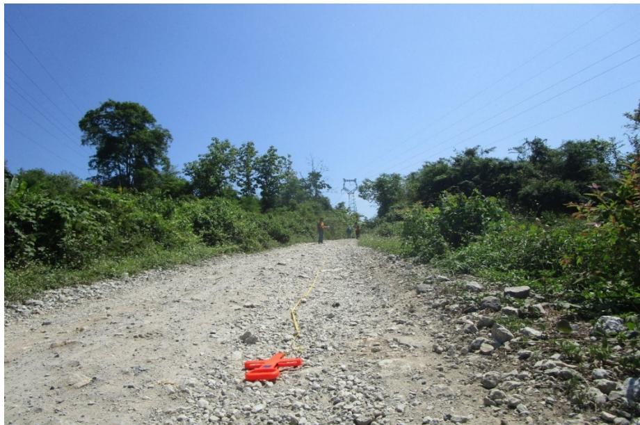
Figure 5. Steep curve section and slope (Km3+850), Local Road No. 2571
