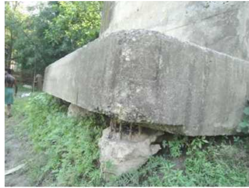
Missing concrete and exposed rebar
