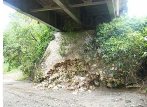
Figure AP 1.20.1 Broken Slope Protection
