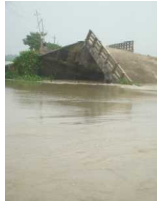
Figure AP 1.13.2 Heavy Bridge Scour
