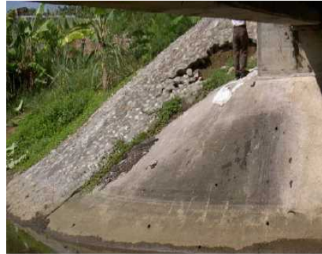
Figure AP 1.22.1 Damaged Slope Protection
