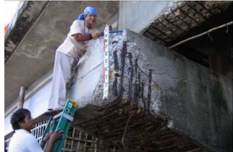
Figure AP 1.5.1 Damaged Pier for Repair by Recasting
