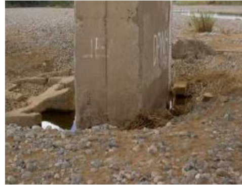
Figure AP 1.21.1 Local Scouring around Pier
