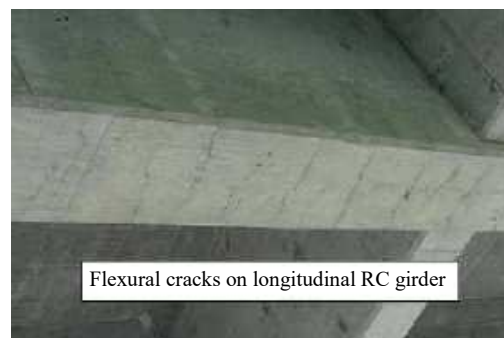
Figure AP 2.2.4 Flexural Cracks at the Center Portion
