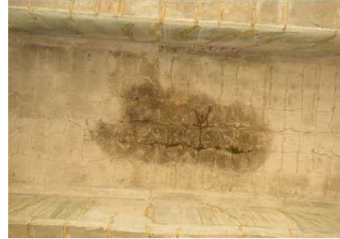
Figure AP 2.6.1 Severely Damaged Deck Slab
