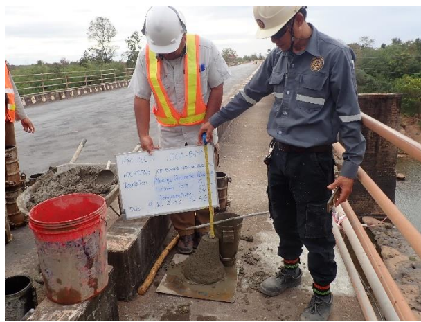
Concrete casting work on 9 th January 2023. Slump test 9.0 cm, Concrete Temperature 34.0 °C
