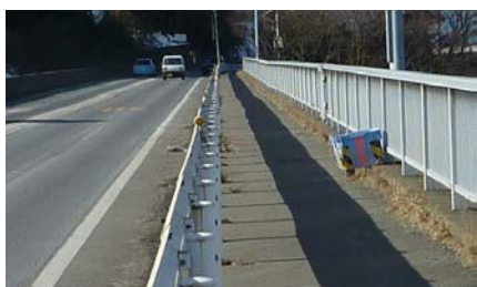
* The photograph shows an abnormal deflection of a bridge with a central hinge.
