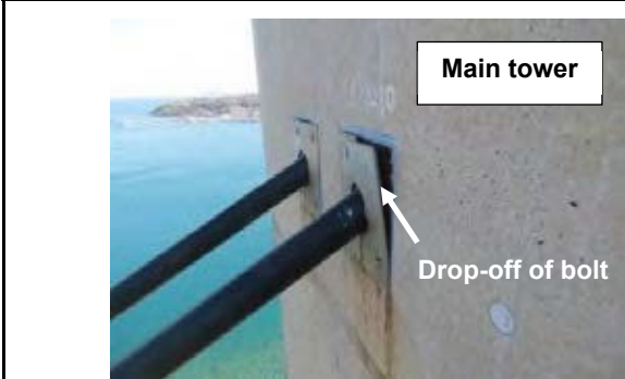
Example of damage to the protective cover of the saddle part
